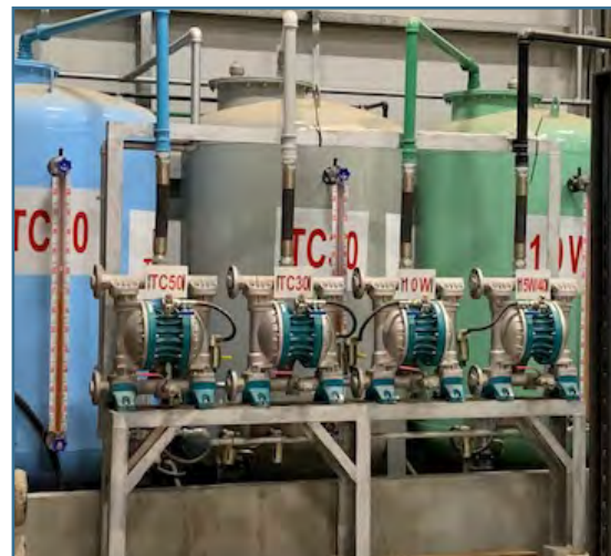
ASTRAevo pumps (1 1/2" metallic version) installed for lubricant transfer (China).
