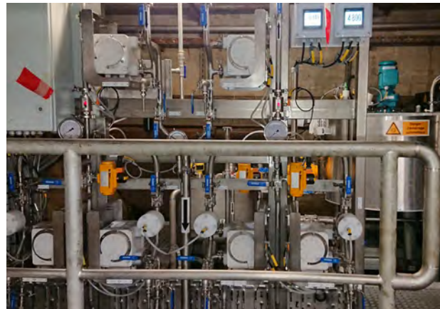
QUANTUM pumps for acid mix transfer (Belgium)
