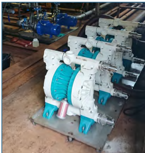
ASTRAevo pumps (1 1/2" PP+glass version) installed for wastewater treatments (Belgium).
